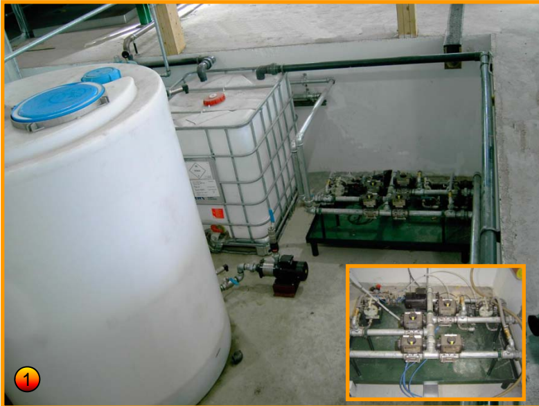
1: Automatic mixing system with piping and filtering.
